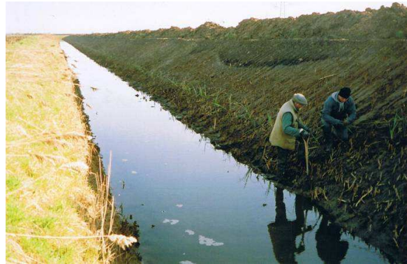
FIGURE 9: Operatives reinstating ‘home-grown’ common reed ( Phragmites ) after an improvement on sewer 3/62 near Friskney
