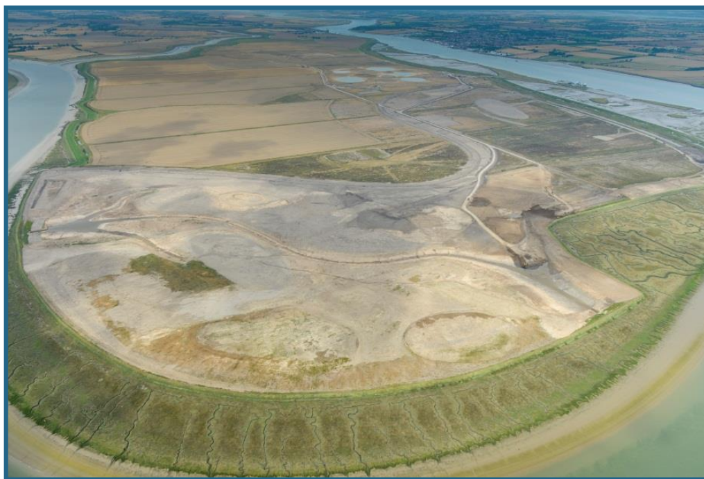
Figure 2.4: Wallasea Island Wild Coast Cell 1 under construction as viewed from south east (August 2014)
