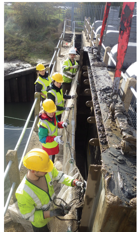
Students from Hull University help attach nets at Hobhole Pumping Station (Martin Redding)
