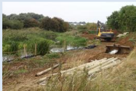
Creating a two-stage channel for improved flood management, September 2013 (Nene Valley). Photo credit: Simon Whitton
